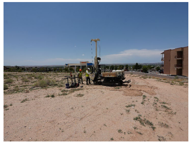
Photo 12: View of dual tube borehole sampling at borehole B-4 at the subject property.
