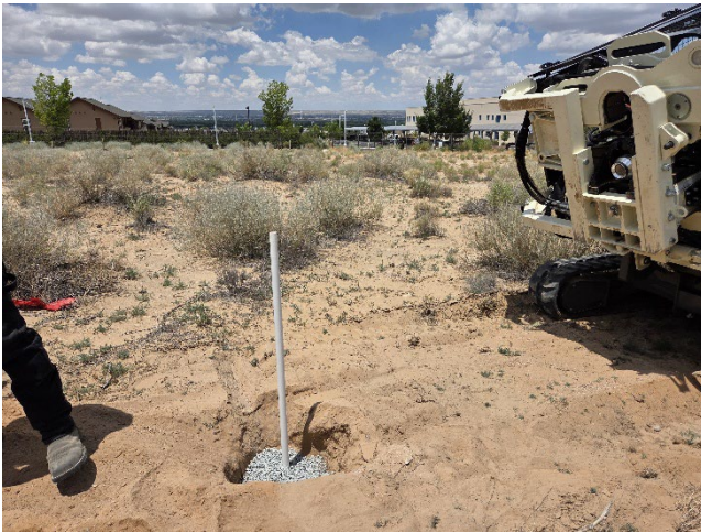
Photo 9: View of installing a temporary landfill gas monitoring point at the subject property.
