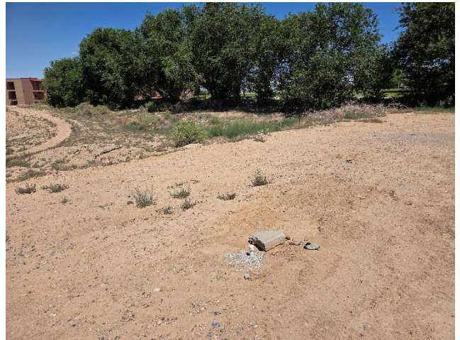
Photo 16: View of LFG-1 capped between monitoring events at the subject property.
